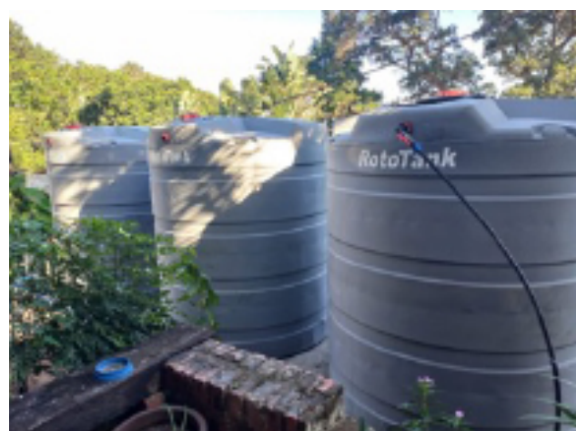
South Coast Hospice installs water tanks to ensure potable water for patients, 2022
